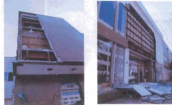
Fall of exterior wall of steel structure (Oroshimachi)
