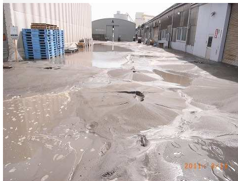
Settlement of nearby ground
