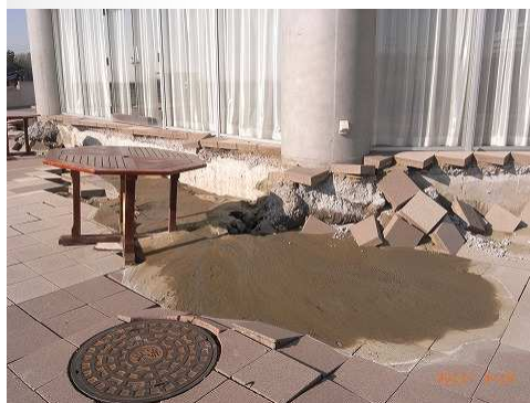
Settlement of nearby ground
